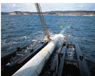
Fig. 1 Photo of undersea pipeline.
